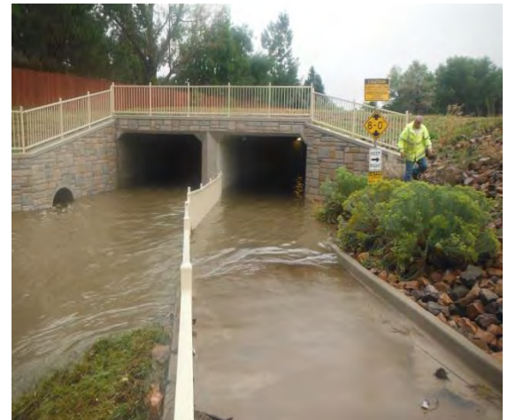
Little Dry Creek @ Arapahoe Road required the pedestrian trail culvert (designed to convey the larger storm event overflows) in addition to the main stream culvert to carry flows during the September storm events
