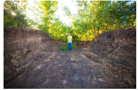
Cherrybrook pond's north embankment breach
