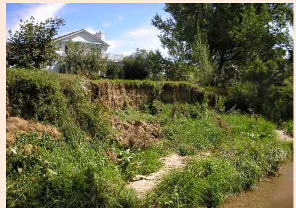
Big Dry Creek channel and bank instability identified in the master plan; this will eventually be addressed with a SEMSWA capital construction project
