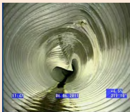
Damaged pipe at Mineral Ave/Vincennes Way
