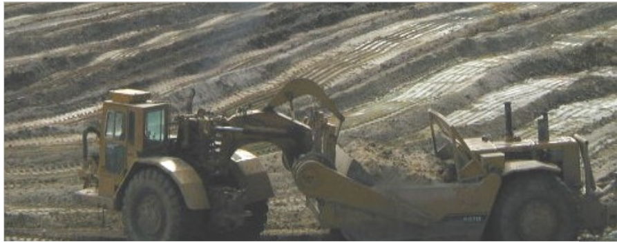
Rates of erosion increase dramatically during construction.
