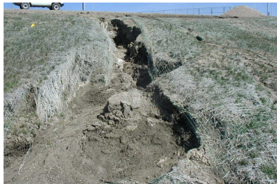
Control of construction site erosion in the City is mandated by Federal and State law.
